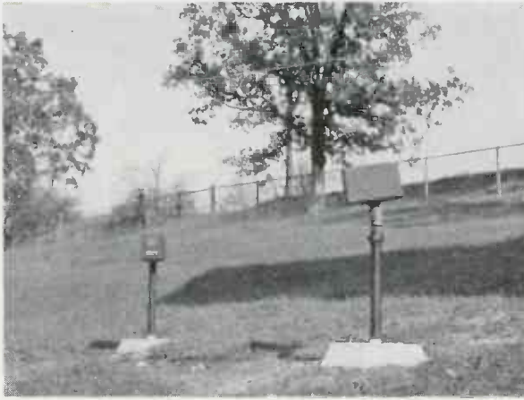
Infra-red photo-cell beam guards station grounds
