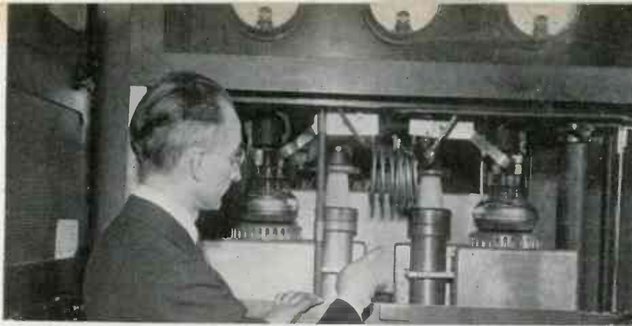
The 50-kw power amplifier unit as installed in panel in main transmitter room. Close-up at right shows unit before installation
