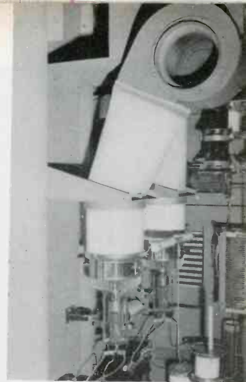
Rear view of final power amplifier, showing blowers
