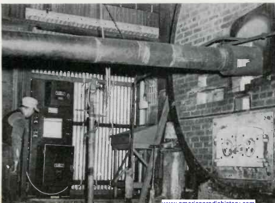
TEMPERATURE control of rotary cement kiln of Lawrence Portland Cement Co., Northampton, Pa. Phototube holder and optical system on standard to left of center in photo. This G-E pyrometer unit has double-chart recorder, amplifying equipment, and speed control contactors mounted in panel
