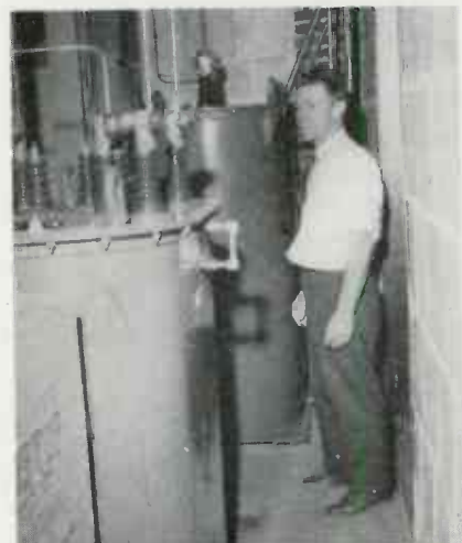
Chief Engineer Valentine with Amertran Class B modulation transformer (foreground) and final power amplifier plate reactor
