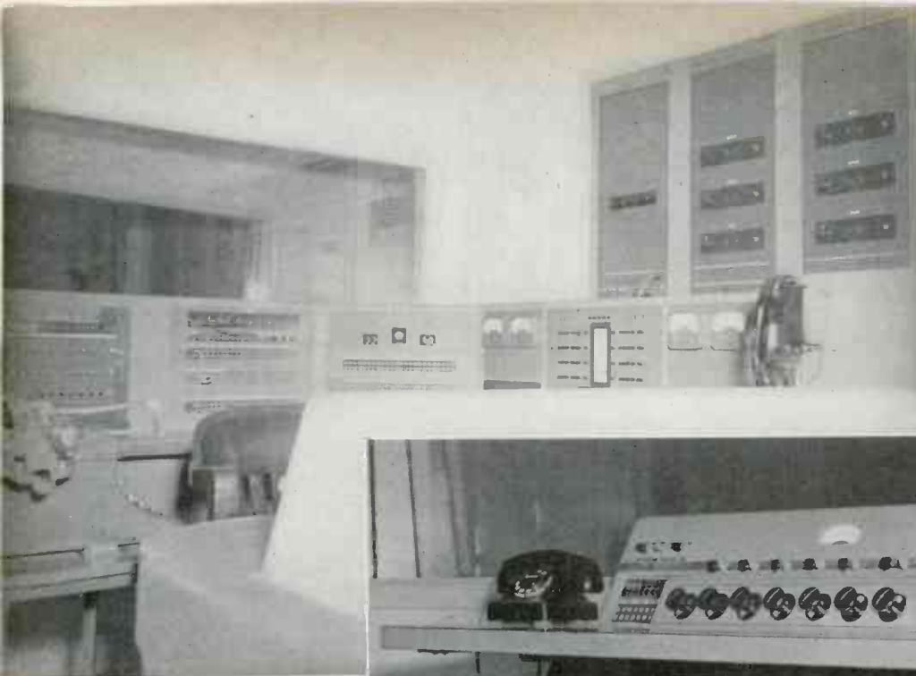
Left—Complete set-up in master control room
